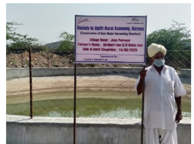
A pond with a capacity of 405 cubic meters has been constructed in Juna Patrasar Village
