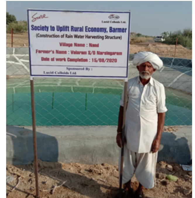
A pond with a capacity of 405 cubic meters has been constructed in Nand Village
